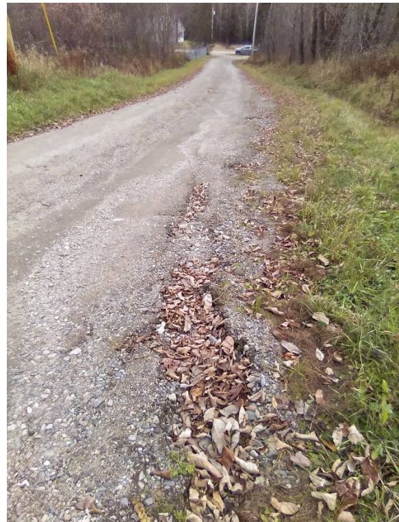
In segment 130995 and 130980, water from the driveway runs along the road surface because it cannot reach the ditch, and the ditch is not stone lined
