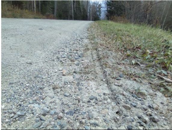
Grader berms, poorly shaped shoulders, and lacking crown cause water to flow along the road surface in all segments
