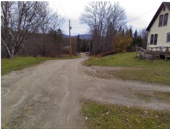
A driveway lacking a cross culvert causes water to run across the road surface in segment 130995
