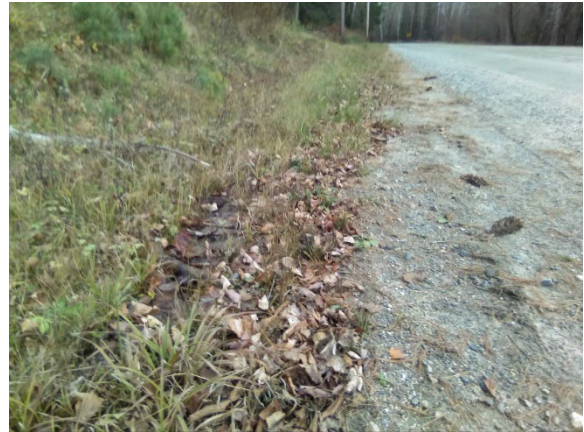
Steep segments lack stone lining in ditches, causing erosion
